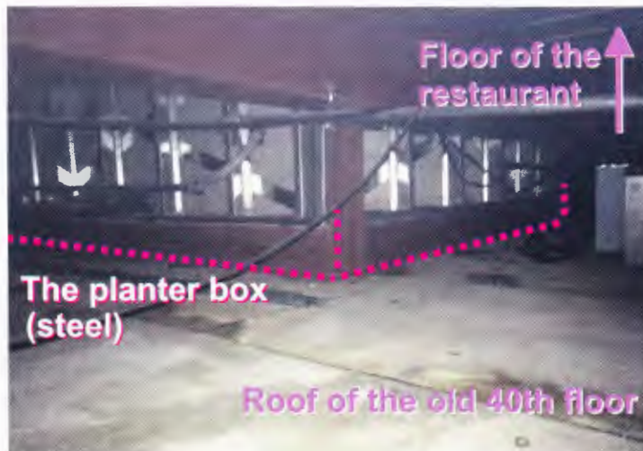
Codit's photo from the crawlspace shows that the steel planter frames weren't much larger than the original 60-inch boxes that the trees were grown in.
