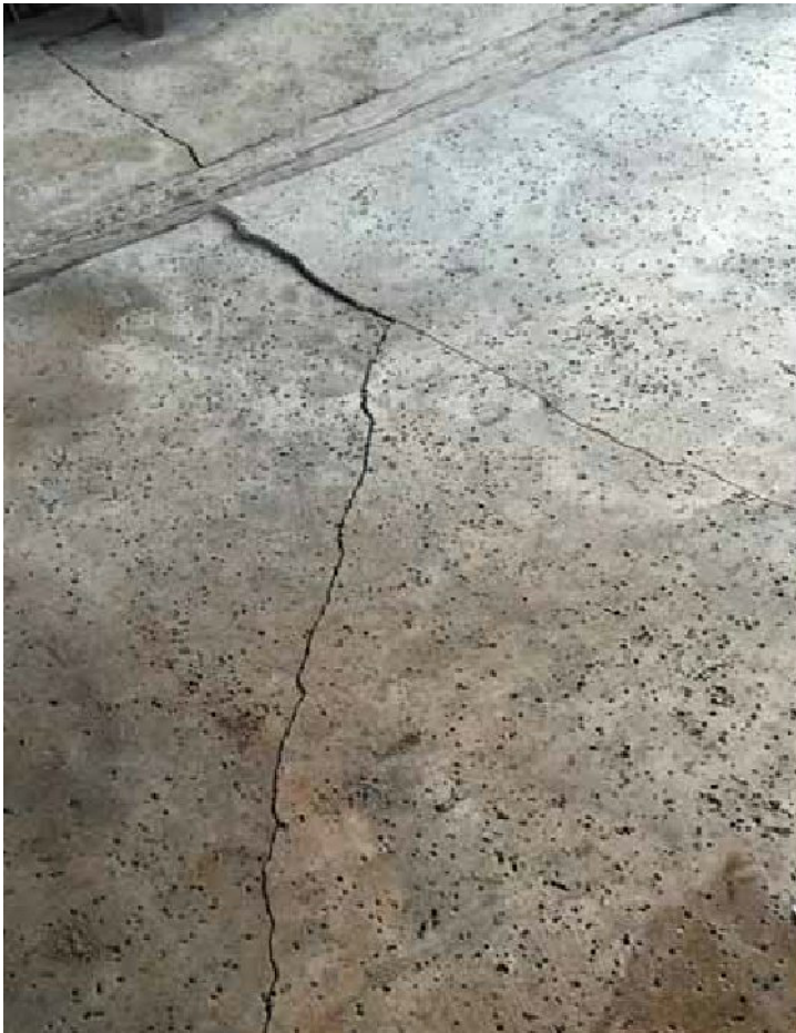
Curious cracks in the concrete out back! Can Dendro close the case?
