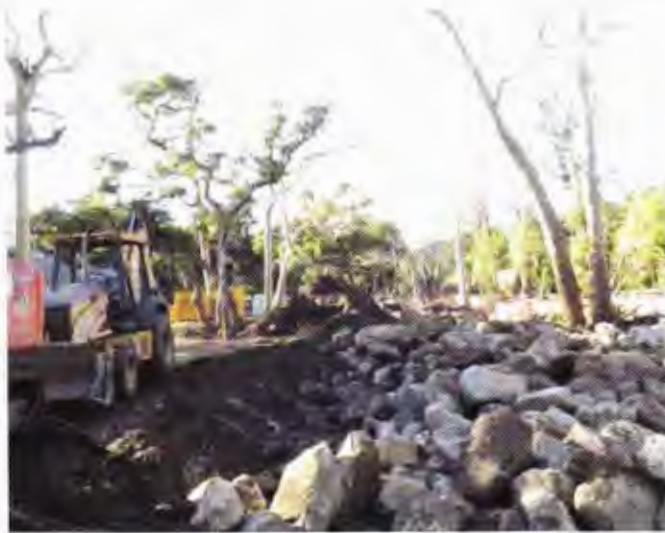
Figure 2. (Above) Post-loss image of a mudslide-damaged property matching the angle of the pre-loss image shown in Fig. 3. All of the boulders were deposited by the mudflow.
