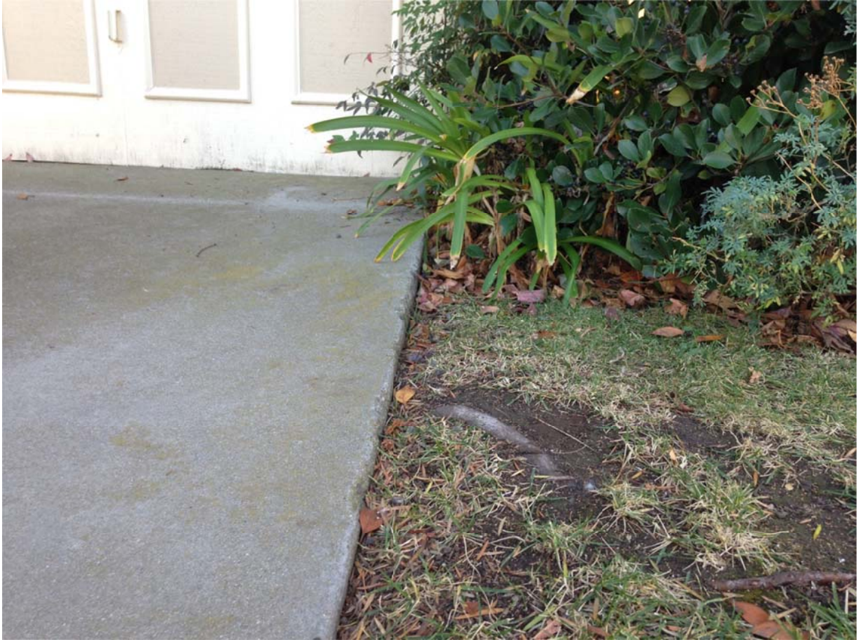
Figure 4: Close up of the displacement in front of the garage door. The displacement of the concrete is approximately 1 inch, making it impossible to open the garage door. The surface root seen at the center of the photo is not likely from the Rhaphiolepis shrub. Rather, this is likely a surface root from the subject Liquidambar tree.
