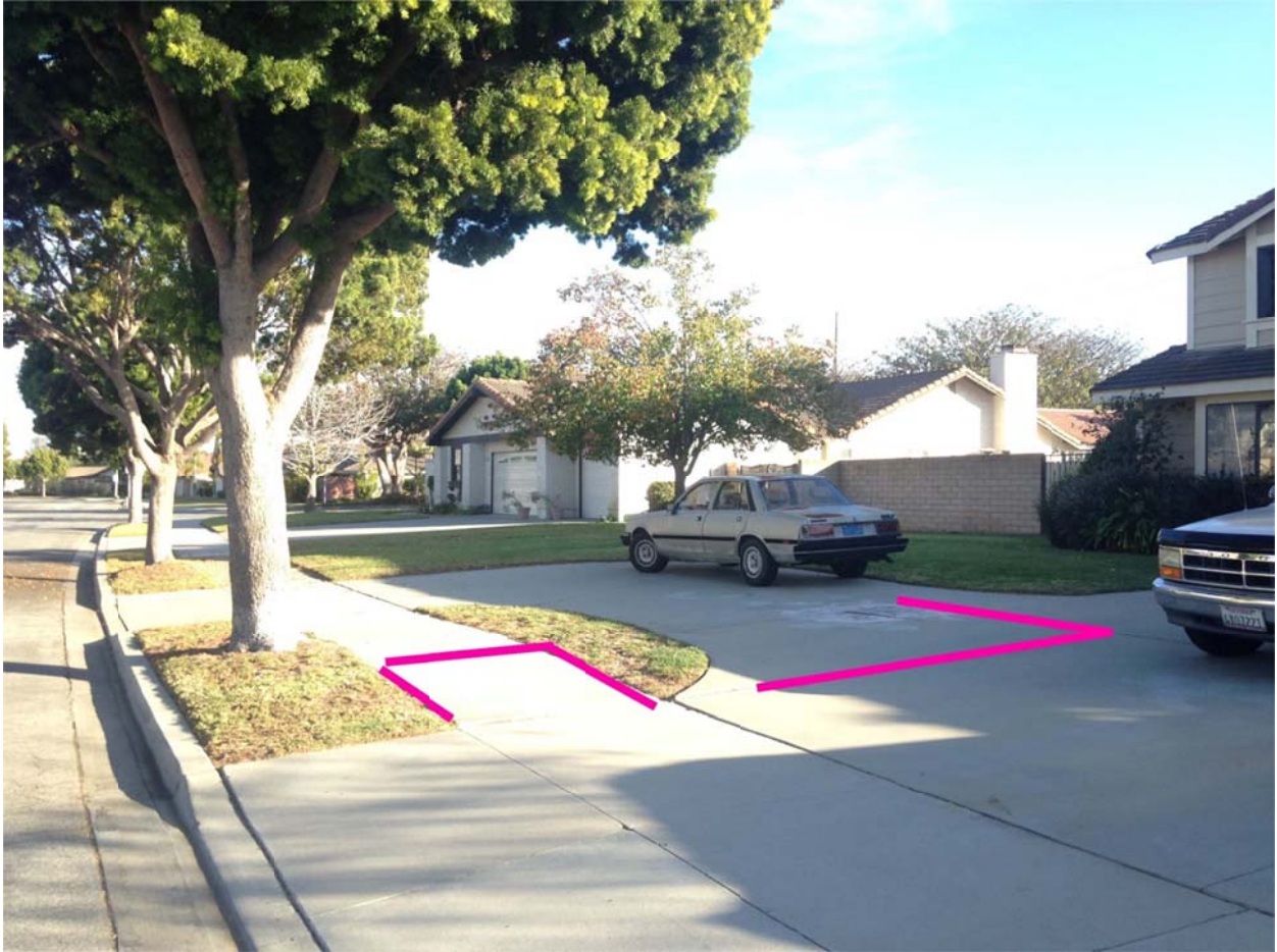
Figure 3: Looking southeast. The next closest tree to the neighbor's driveway is the Afrocarpus tree (left) growing in the street median. It appears to be causing the concrete displacement highlighted in magenta.
