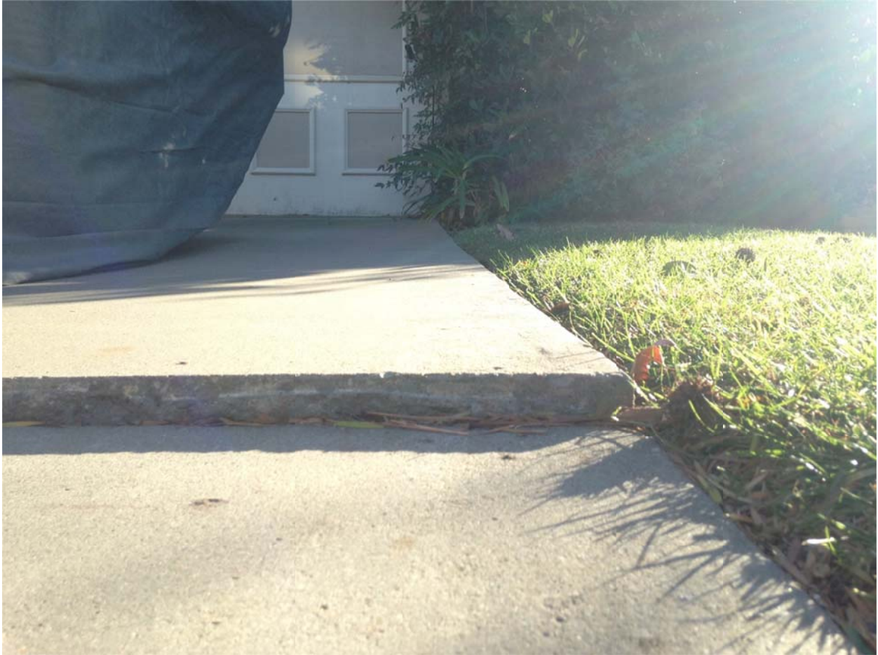
Figure 5: Close up on the displacement towards the middle of the western portion of the driveway. The displacement is approximately 1.5 inches.
